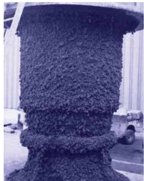
Mussels attached to Pump Shroud
